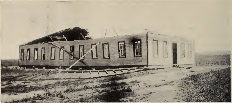
The Boys' Dormitory at Tex.-Mex., after the storm of August 18. This is only a sample of what the storm did to Tex. Mex. The "San Antonio Building" was also unroofed, walls crushed in and floor moved off the foundations. Every other building of the institution was more or less damaged; the two windmills were smashed, the tower and pressure tank taken away. Mr. Skinner is "up against it,"—and just as school was about to open. It will take $2,000.00 at once to put in necessary repairs for resumption of this school's noble work.
